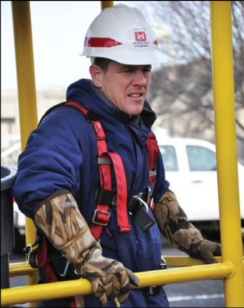
Deputy District Engineer Alan Feistner prepares to be lowered by a crane to the base of Ice Harbor's fish ladder in a man bucket.
